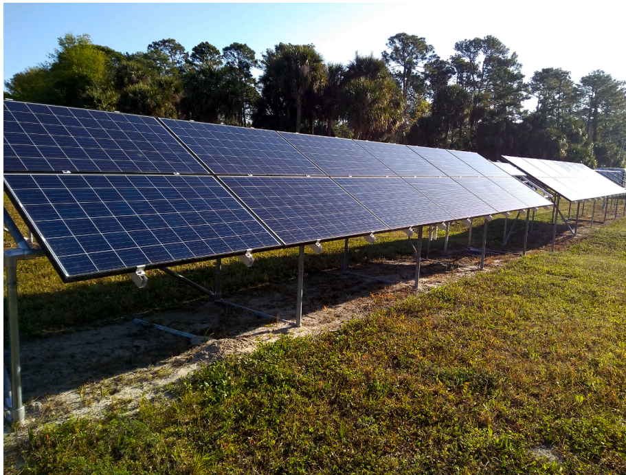
Fig. 1. The two string, grid-tied 6.2kW experiment array at the UCF FSEC test field in Cocoa, Florida.
